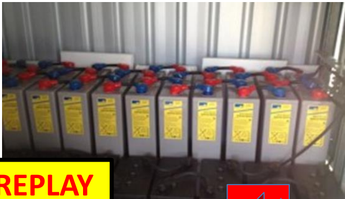
Common stand alone system battery bank
